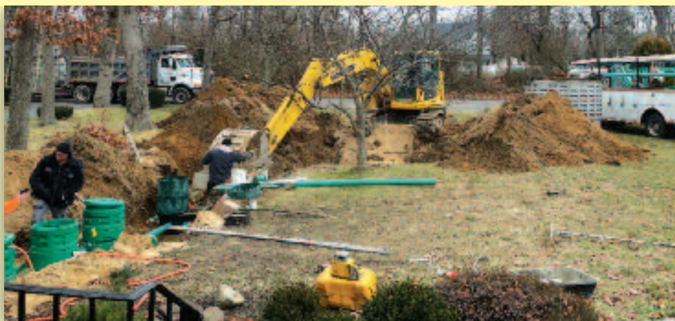
BIG DIGS: Installation of an innovative septic system at a Suffolk County home.
