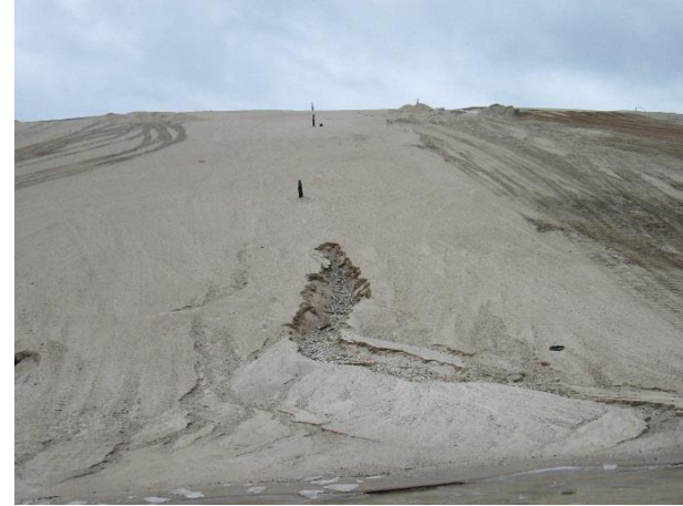
Side Slopes: View after washout of sand layer after a major rain event that plagued the cap project during the construction period
