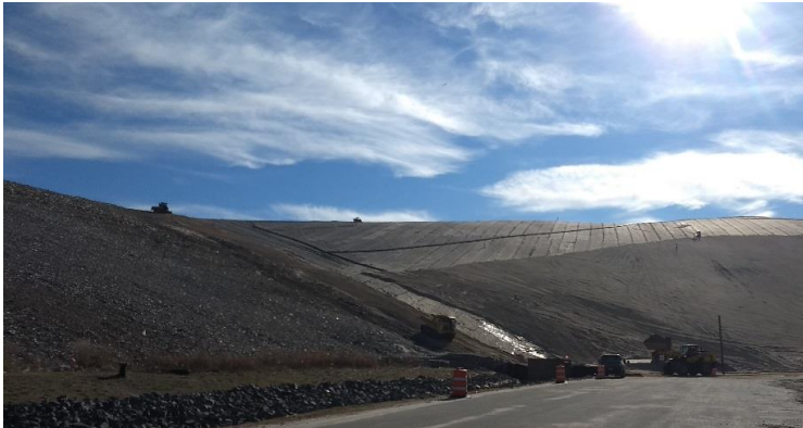
View of the barrier protection layer: using fresh sand to replace sand that was washed out by rain
