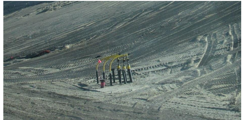
Upgraded horizontal gas collection headers connected to horizontal gas collection pipes at various elevations of the waste mass
