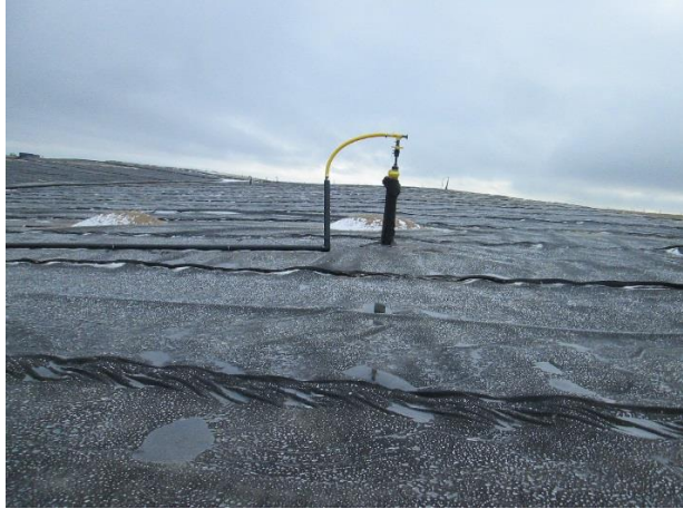
Vertical Gas Extraction Well: View of a completed gas extraction well after hook-up to the gas header pipes connected to the landfill gas flare system
